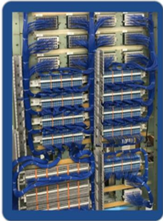
Railway Signalling Panel
